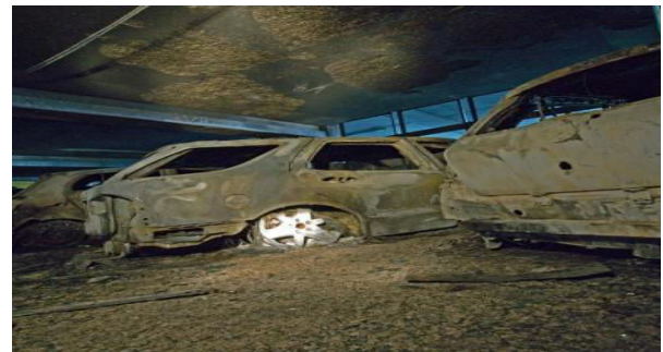
Figure: Surface spalling after a fire in a car park
