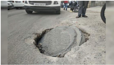
Figure 2. Broken Manhole Cover
