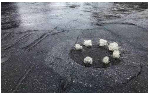
Figure 3. Overflow of water from manholes
